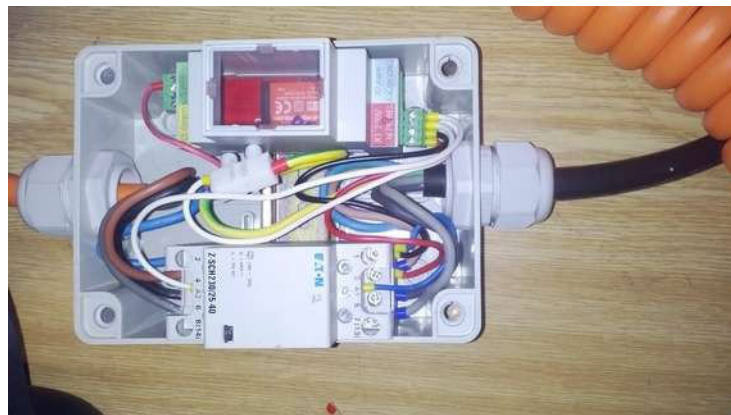
Picture 18: Charging cable made with EVSE DIN together with 4pole contactor in a box
